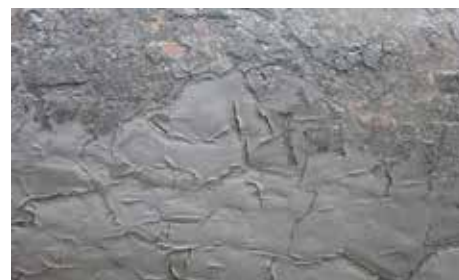
Tar and rust before blasting
