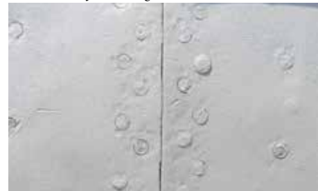
The same spot revealing bare steel after 94 years
